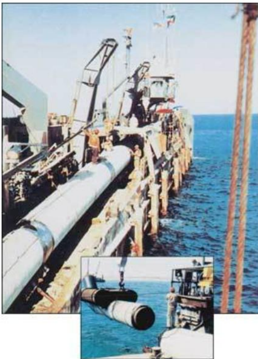
Figuur 28 Pipeline operations under way in the early 1960s aboard Brown & Root's lay barge L.E. Minor. Inset illustrates how weighted pipe is handled before welding it into the line. (Courtesy of Halliburton)
